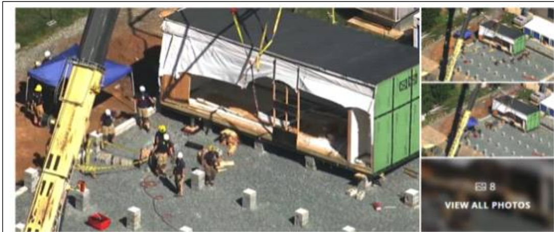
A deadly construction accident has been reported at Heights School in Potomac, MD. Thursday, Aug. 23, 2018. (SkyTrak7)
